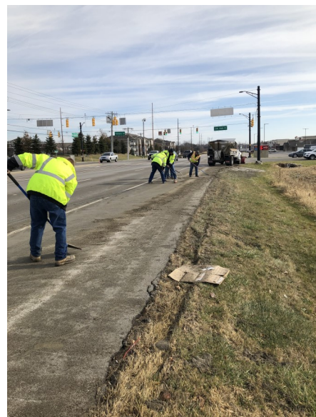
Emergency response by street department to clean up concrete spill on Whitestown Parkway
