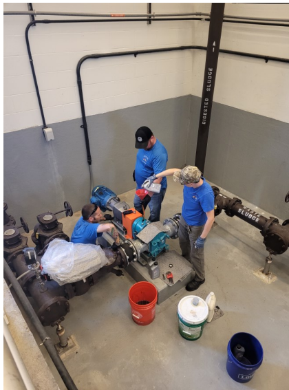
Changing oil in sludge feed pump
