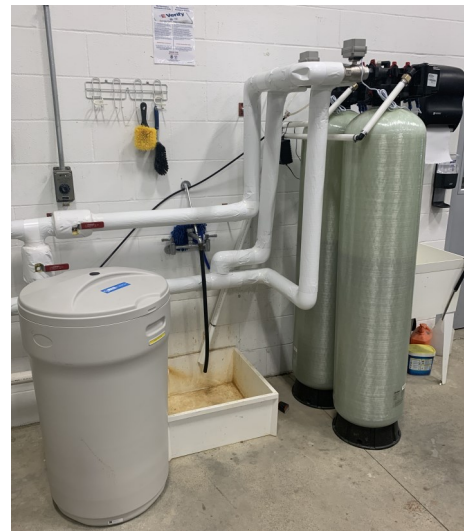
WATER SOFTENER FOR ODOR CONTROL AT THE WASTEWATER TREATMENT PLANT
