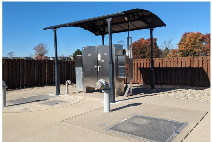
NEW CANOPY OVER CONTROL PANEL LOCATED IN GOLF CLUB OF INDIANA LIFT STATION
