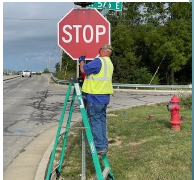
New Stop Sign and Blinkers at 575E and ASW
