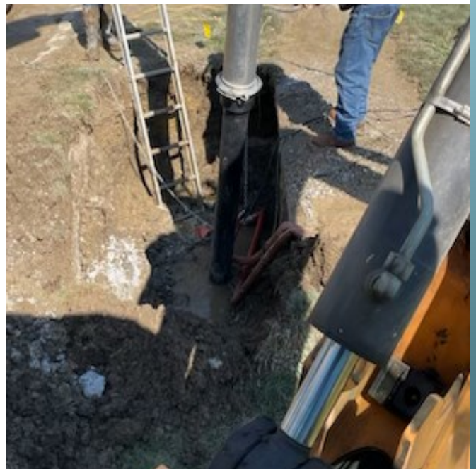
Water Main Break in Royal Run
