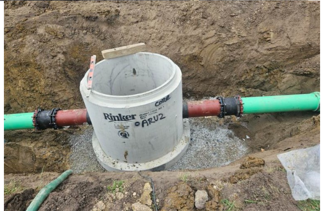
INSTALLING AN AIR RELIEF VALVE FOR THE NEW FORCE MAIN AT PEABODY
