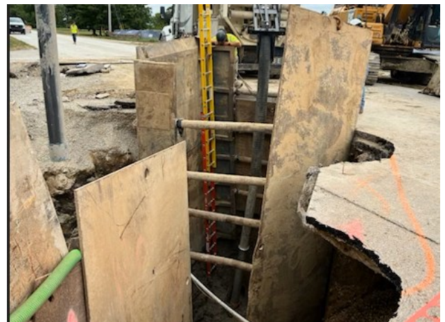
SANITARY INSTALL FOR SOLSTICE APARTMENTS
